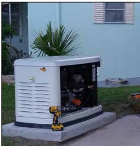
The generator by the office
